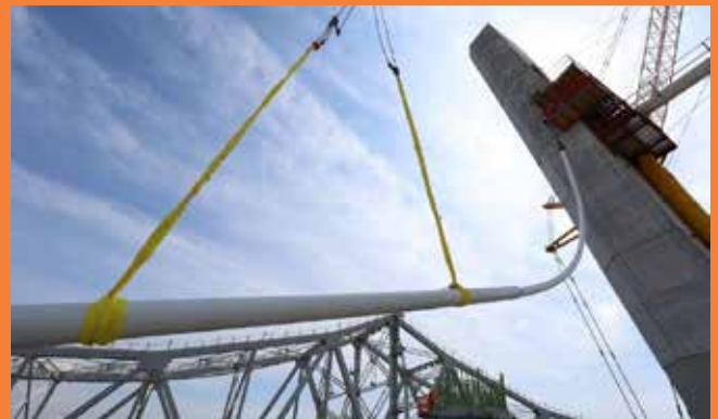
▲ A crane hoists the cable to its anchorage within the 272-foot tower of the new Goethals Bridge. Photograph courtesy of Mike Dombrowski, Port Authority
