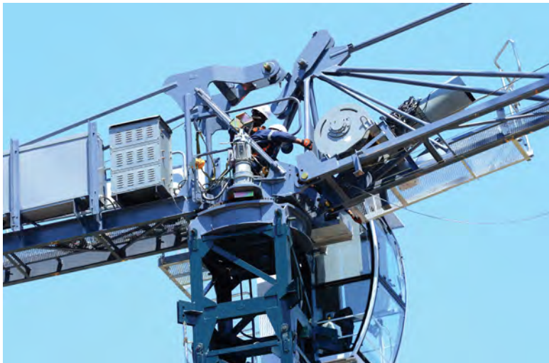
The jib foot being connected to the slew turret during crane erection.
