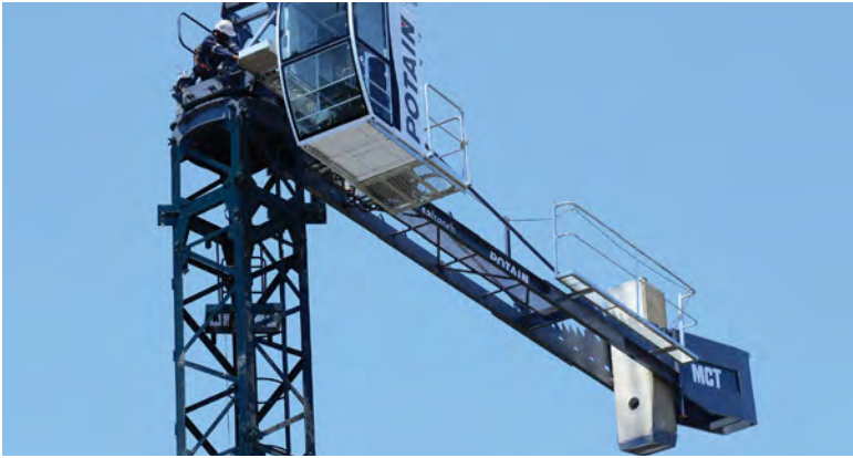
The state-of-the-art Potain cab being positioned on the tower crane during the erection process.
