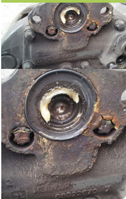
Adjusting and clamping mechanisms corrosion
