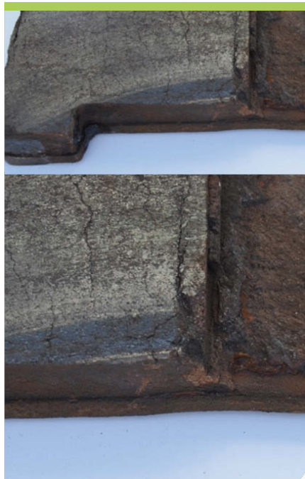
Partial or full separation due to mechanical reasons
