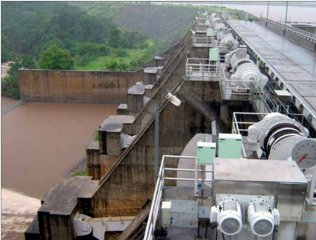
Kapichira hydropower station in Malawi generates 64 MW of electricity, and there are plans to double the output.
