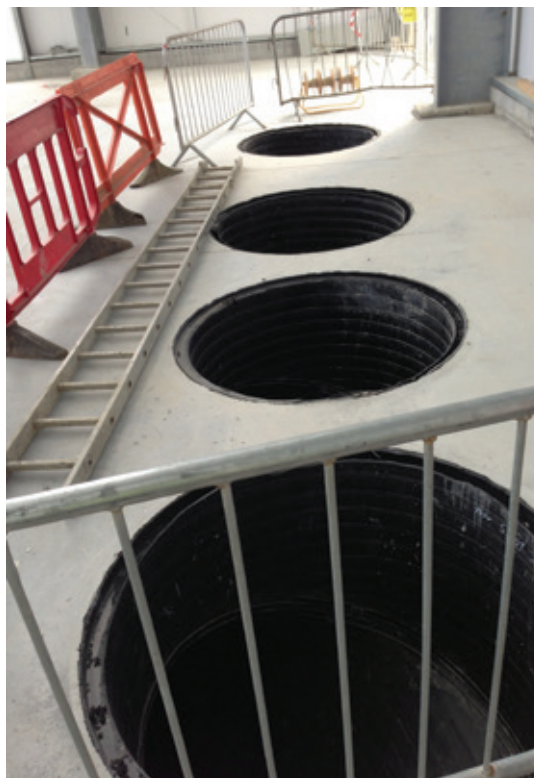
Asset supplied 750m of Weholite pipe for the network of underground pipes
