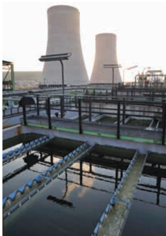
The Sasol Landlord project is a zero liquid discharge (ZLD) plant, where water with concentrated salts is treated in different streams at the highest-quality level.
