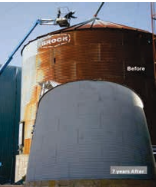
A before and after image of the BMG Rust-Anode cold galvanisation system, which was applied to galvanised sheeting to extend its life.
