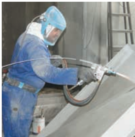
Thermal sprayed aluminium (TSA) being applied to a footbridge using the flamespray process.
