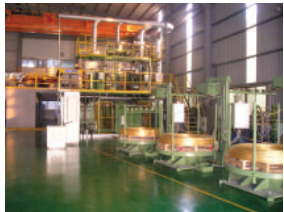
▲ Continuous casting plant from Rautomead of Scotland
