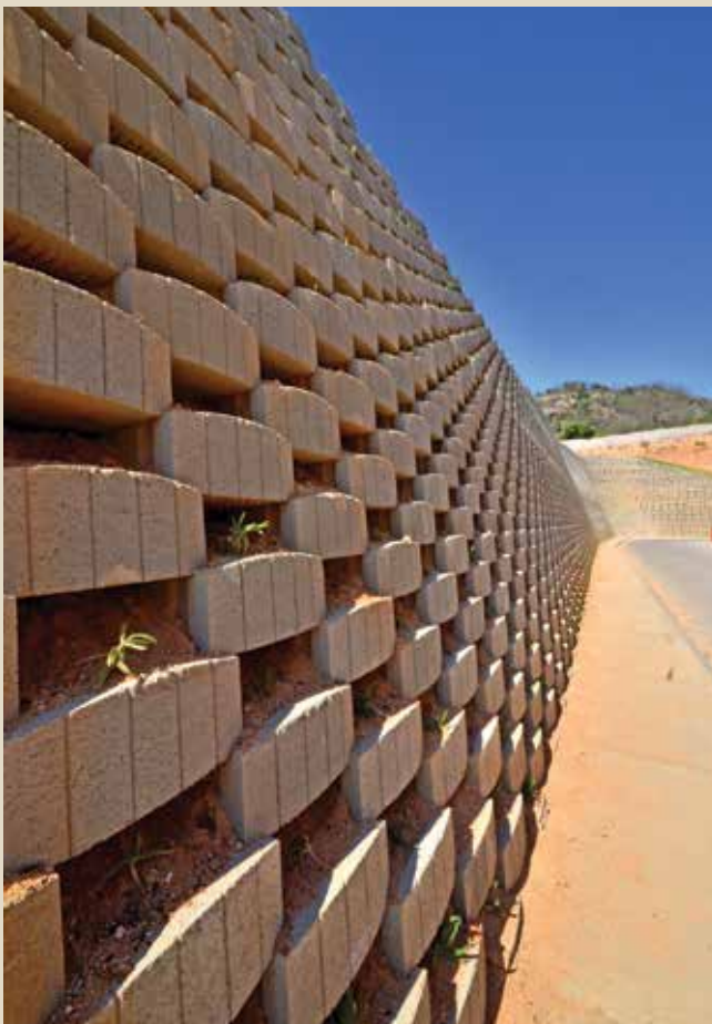
The 200 m perimeter wall built with Aveng Infraset's TB 490 and TB 300 concrete retaining blocks.
