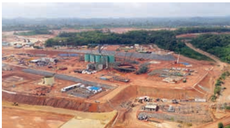
Aerial view of the Asanko Phase 1 site, where construction has now passed the 60 % point (photo: Asanko Gold).
