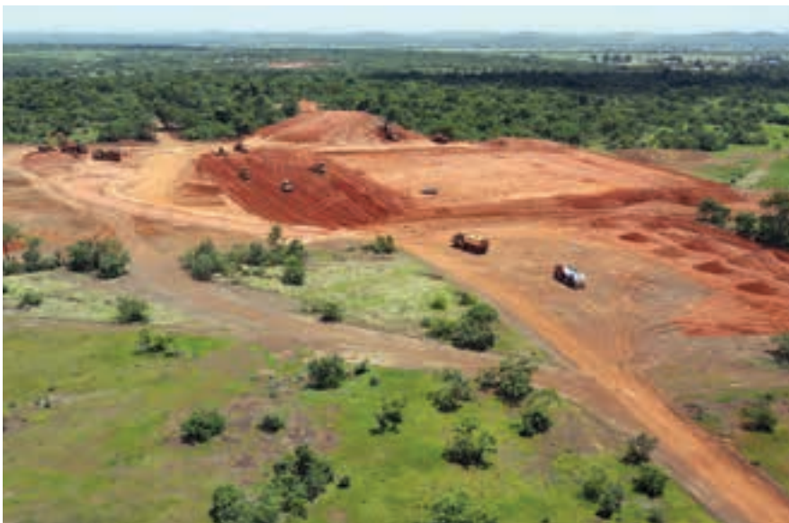
Earthworks in progress at the Yanfolila gold project site in Mali (photo: Hummingbird Resources).
