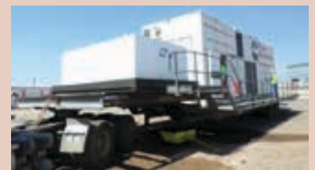
Cummins has reconditioned a 2 MVA Cummins motivator for Debswana's Jwaneng mine.
