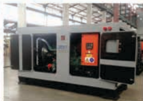
Diesel generator set housed in a sound attenuated container
