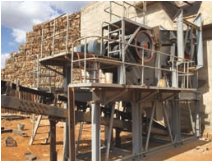
The primary crusher at Pickstone-Peerless, which has now been commissioned (photo: Vast).
