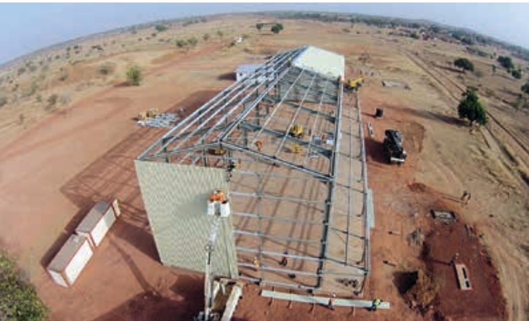
Construction underway at Karma late last year. The site has progressed considerably since then (photo: True Gold).
