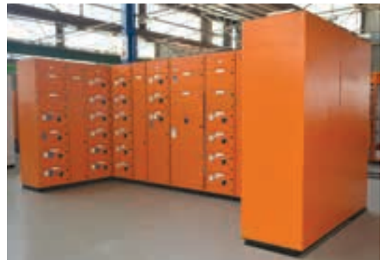
A fixed pattern MCC manufactured by Shaw Controls for an E-house destined for a mine tailings project. "There is no other manufacturer in the country that is able to manufacture everything in-house," says Van Niekerk.
