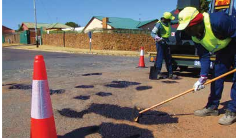
Repairs being carried out using hot mix in a bag which is being specified as an approved and effective alternative to conventional, bulk hot mix asphalt by consulting engineers.
