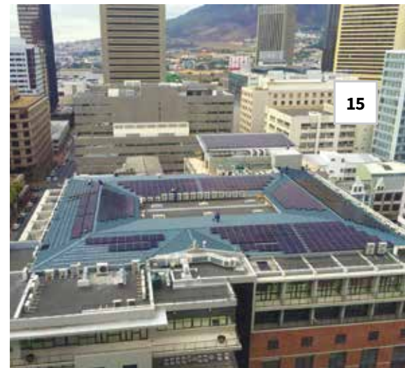
The 103 kWp 33 Bree Street project.
