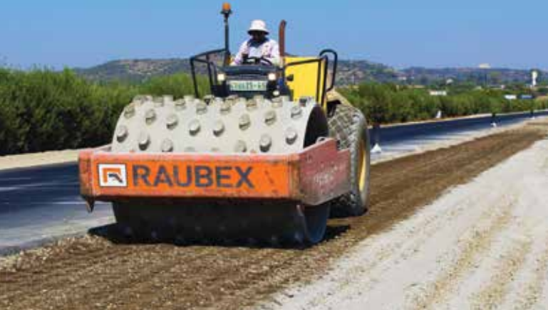
Raubex is stabilising the sub-base to a depth of 350 mm with AfriSam's Roadstab 32.5N CEM ii B-L cement.
