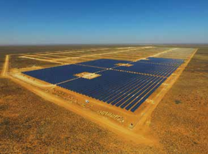
Aerial view of a portion of the Mulilo-Sonnedix-Prieska PV project, a 125 hectare solar PV project valued at R1,3-billion and situated 50 km south-west of Prieska in the Northern Cape.
