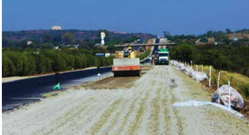
Some 20 000 tons of AfriSam's Roadstab 32.5N CEM ii B-L cement will be used on this project.
