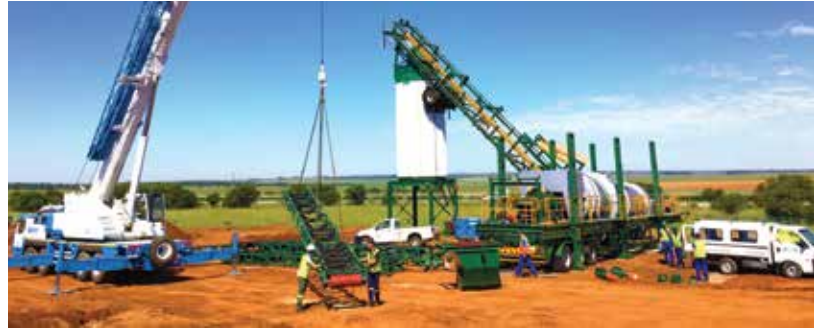
Actop Asphalt's second Comar continuous mix plant, with its high 120 t/h continuous mix capacity, is also capable of handling 40% recycled asphalt (RA).
