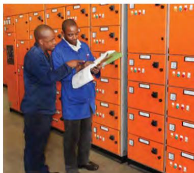
The Rockwell Automation and JB Switchgear Solutions collaboration provides a cost-effective, high-performance technical solution.
