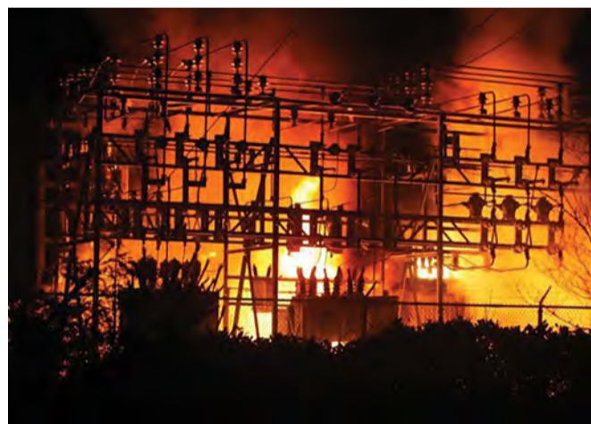
Substation fires usually take thousands of litres of water and hours to extinguish.
