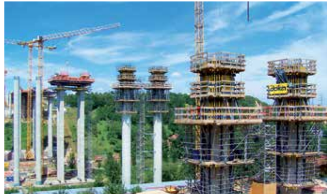
Pairs of super-slim reinforced columns carry the superstructure. The diameter is no more than 2,80 m at the widest and the highest piers are 57 m tall.
