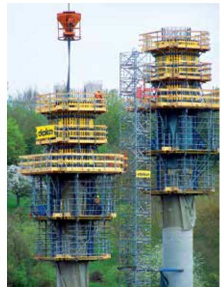
The formwork for the circular-section primary piers climbs with Automatic climbing formwork Xclimb 60. Guiding shoes hold the system locked against the structure at all times.
