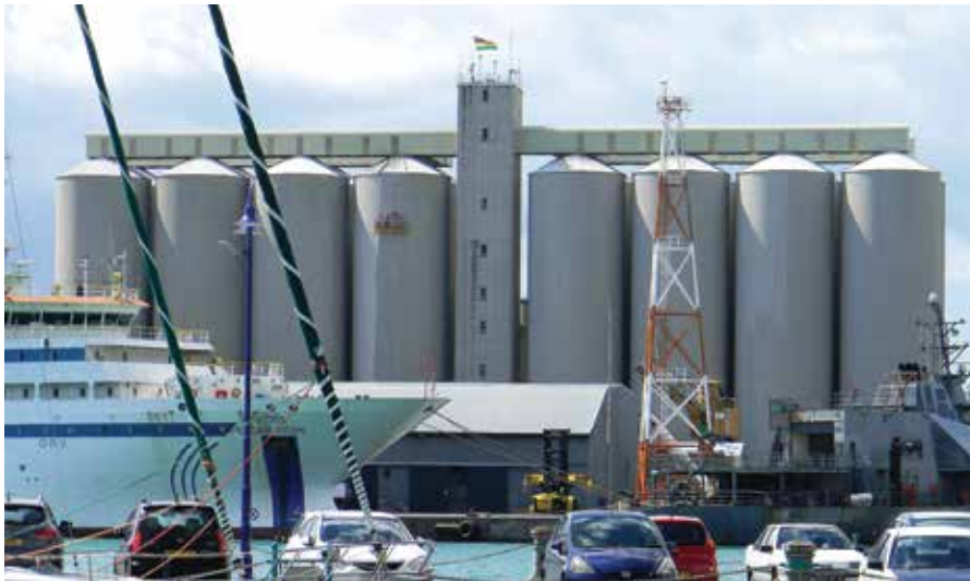
Work in progress applying a.b.e. protection near the top of the towering wheat silos in the Port Louis harbour, and the fully repaired structures which are a focal point of the ocean gateway to Mauritius.
