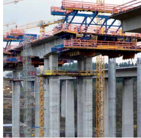
Doka supplied four cantilever forming travellers with four longitudinal trusses per carriage for building the superstructure of the Lahntal viaduct. Complete with formwork and platforms, each cantilever forming traveller weighs about 130 metric tons.
