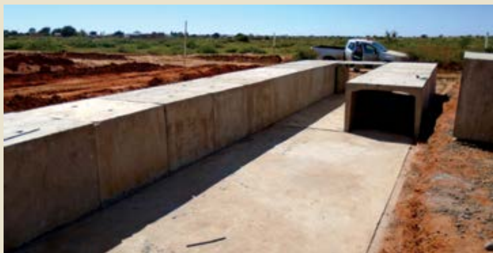
BELOW: Installation of precast culverts, part of the appurtenant works associated with the contract.
