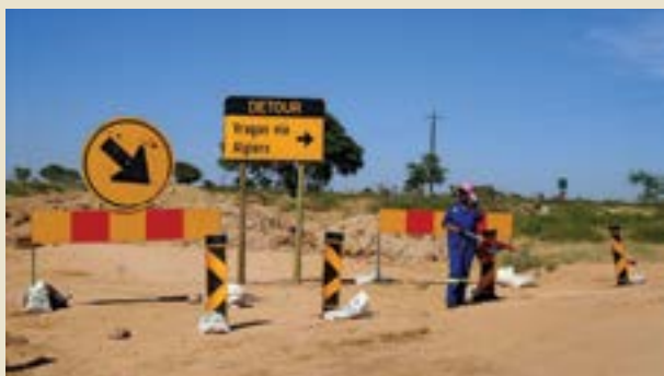
Traffic accommodation in the construction area. The location is about 70 km north of Vryburg.
