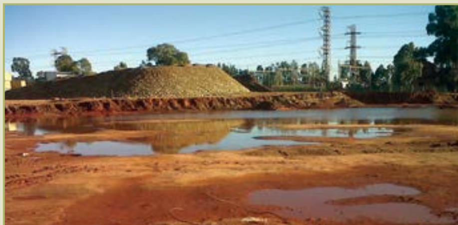
Heavy rains and a mix of in-situ material rendered conventional reinforcing methods ineffective.
