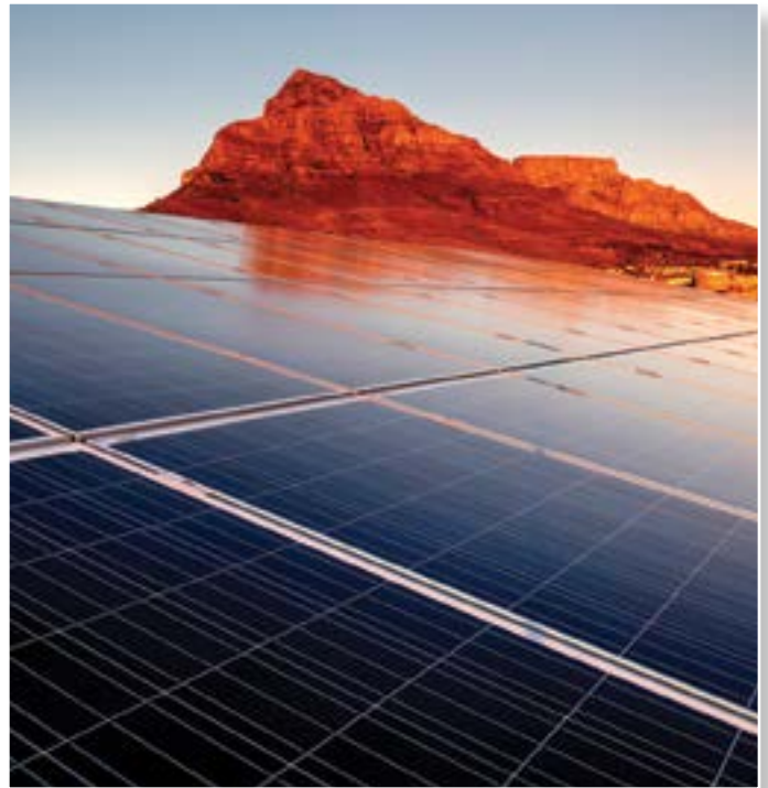
The 1.2 MW Black River Park Solar Project has broken new ground in becoming the largest integrated PV plant in Africa and the first to legally transmit electricity back into the City of Cape Town's electrical distribution network.
