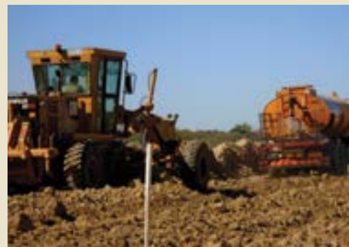
ABOVE LEFT AND RIGHT: A load-and-haul operation to produce fill material for Murray & Roberts Infrastructure's contract to upgrade various gravel roads in the Ganyesa area of North West Province; Filling a water cart at a water point. Other equipment on-site includes graders, rollers, tipper trucks, excavators and TLBs.
