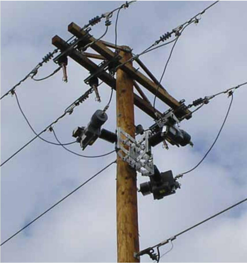
Photos courtesy of Blue Grass Energy
