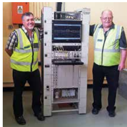
ACTOM Signalling's Frans Badenhorst (left), Application Engineer, and Leon Pienaar, Senior Development Engineer, with the newly-installed electronic interlocking system in Crescent station's relay room.
