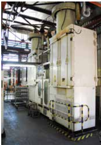
Figure 3: Existing impregnation machine (photograph taken at Robert Bosch Production Plant, Brits).
