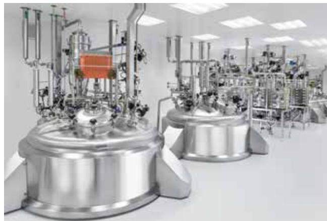
Figure 3: Application example in the chemical industry. (Image courtesy @werbefoto-burger.ch).
