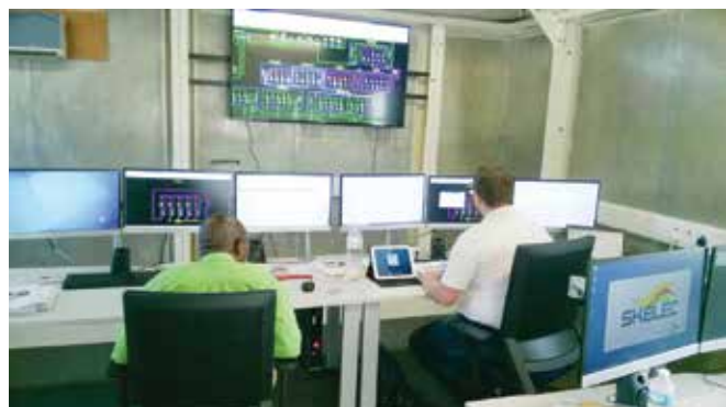
Figure 3: Control room displays.
