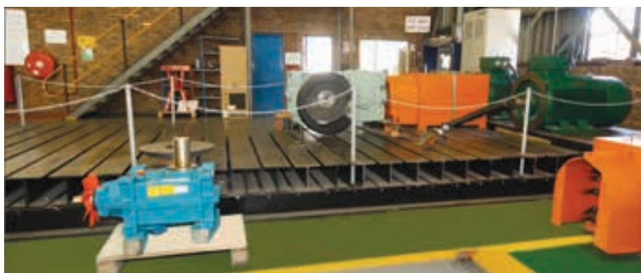
HTSA's new load test bay consists of two VSD-controlled 200 kW induction motors that can operate at speeds from 200 to 3 000 rpm, allowing a large range of operating speeds to be simulated on the test bay.
