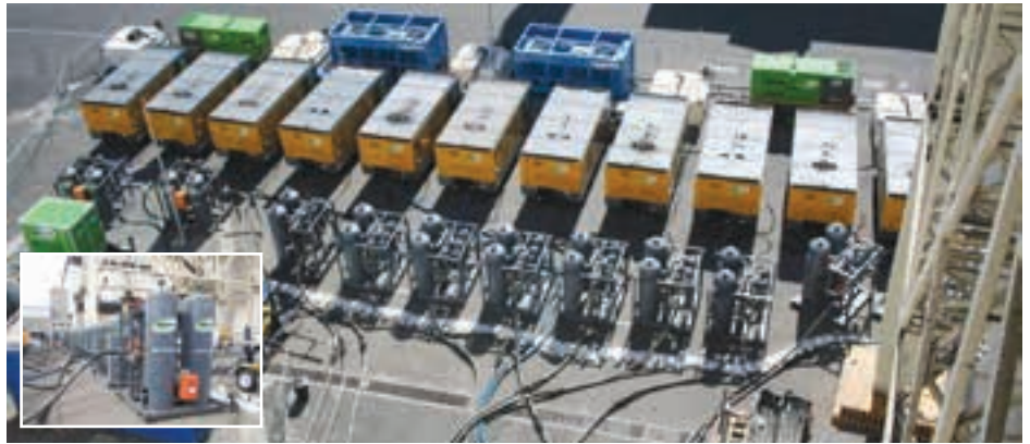
An overview of the pressure-testing project recently completed with Rand Air at the Koeberg Power Station. Inset: Ten PTS916 Rand-Air units running through desiccant dryers pumped dry oil-free air into the containment building.
