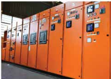
SC100 Motor Control Centre
