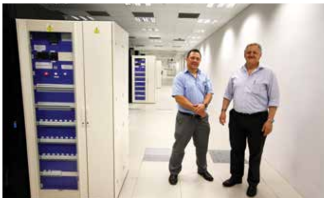
William Blackbeard (left) and Neil van Blerk in one of Vodacom's new data centre halls, which are illuminated by recessed high performance T5 light fittings, controlled by individually fitted passive infrared occupancy sensors.
