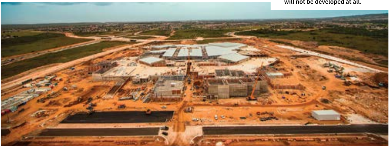
The developers of Baywest City in Port Elizabeth have announced a landmark deal with Vodacom which will see the communications giant install Baywest's fibre optic network, giving high speed internet access throughout the development
