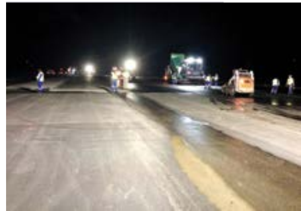
Asphalt surfacing during Phase I of the project, which involved reprofiling of the runway.
