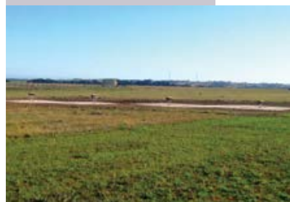
The four Precision Approach Path Indicators (PAPI) at Runway 29, installed by ADB Electrical.
