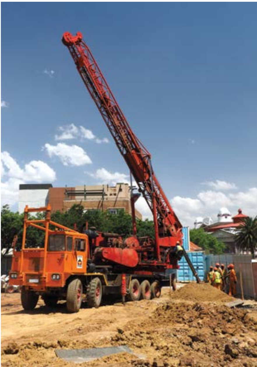
Gauteng Piling providing the foundations for the new City Lodge Hotel in Newtown Junction.
