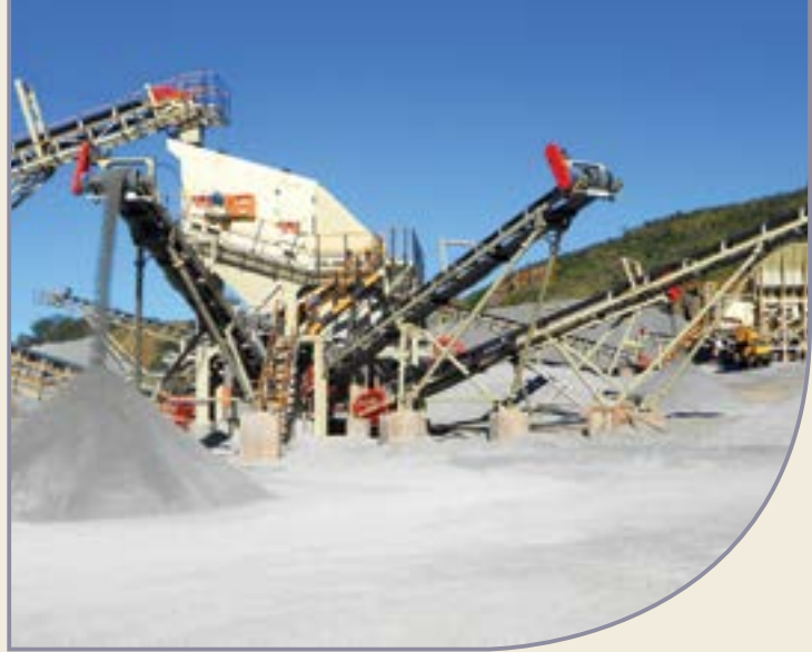
The crushing plant supplied to a Queenstown operation comprises a Metso C100 jaw crusher with a vibrating grizzly feeder, a three deck CVB 1845-3 screen, a four deck CVB 1845-4 screen and two HP 200 cone crushers.
