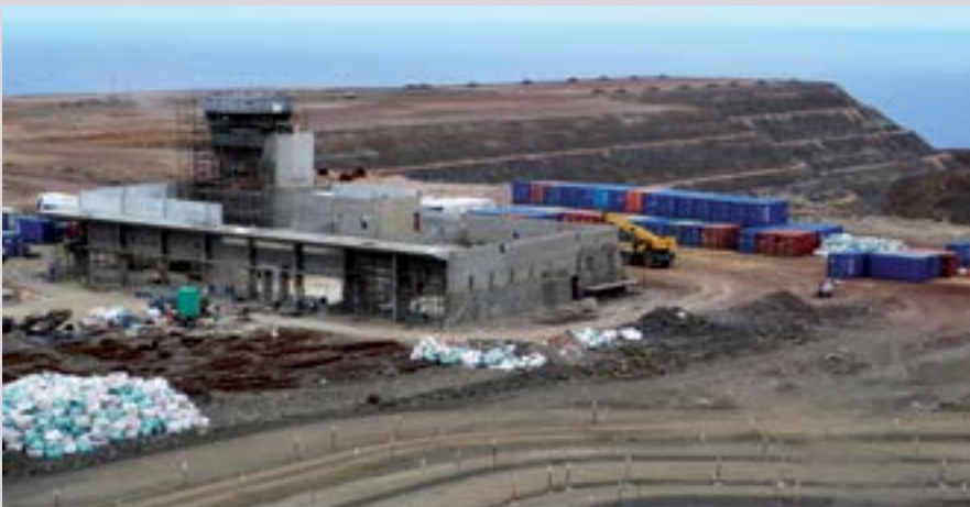
Concrete was specified for the airport runway, terminal building, air traffic control building, fire department building and permanent wharf.
