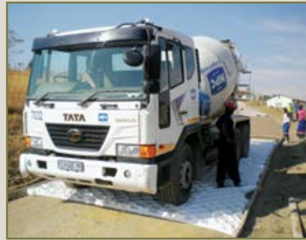
Application is simple: a section of geocell road being filled with concrete.
