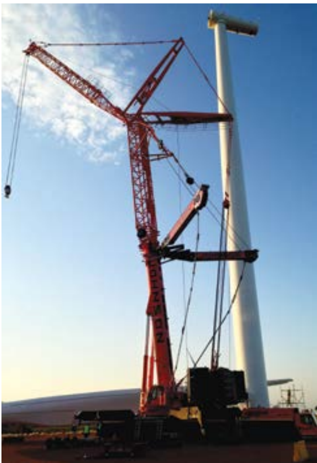
The crane was configured with a main boom of 49,1 m, an insert of 19 m and a 28 m luffing section, totalling 96,1 m, allowing for a hook height of 90,19 m.
