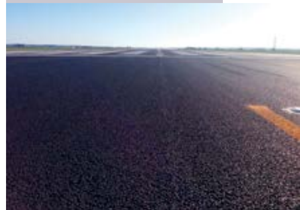
A closer view of the UTFC (Ultra Thin Friction Course) milled and replaced at Runway 29.
