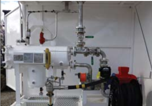
This system has filtration at high flow in and out to refill an on-airport refuelling vehicle.
