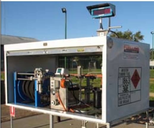
System with closed circuit test, millipore sampling point and high visibility digital register.
