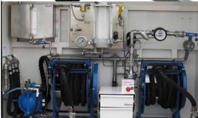
Operating equipment showing delivery and suction reels, air-operated diaphragm pump, closed circuit test system, product reversing valves.
