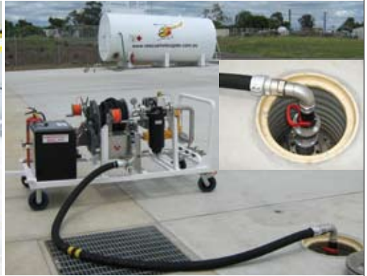
Shows hydrant cart connected to fuel supply in pit.
