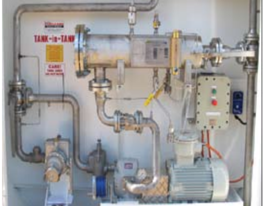
System with variable speed drive to pump with high flow filtration into storage and out to delivery nozzles.
