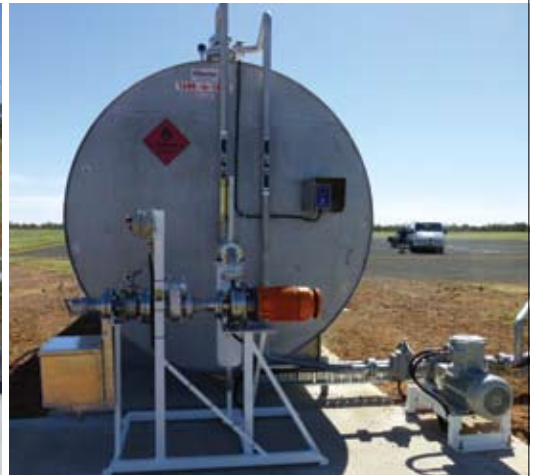
Tank infill and dispensing pumps. Fitted with filtration, pressure differential gauge, emergency stop.
