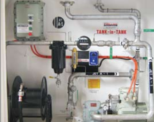
System with variable speed drive to accommodate both over an single point refuelling nozzles.
