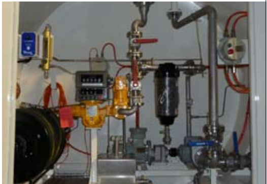
This system with over and under wing refuelling & completely powered by a 3 phase genset.
