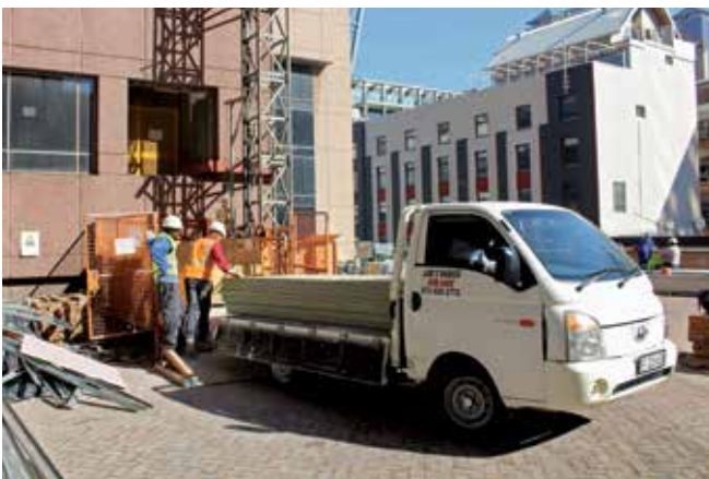
Materials are delivered to the various sites by a hoist that was installed by Murray & Roberts Western Cape.
