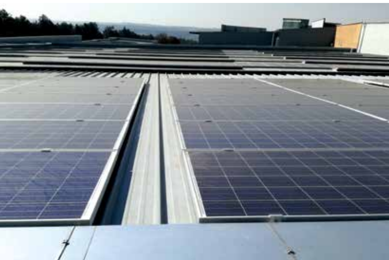
Solareff uses 10 mm Band-It stainless steel band-and-buckle and a C001 tensioning and clamping tool for cable bundling on solar panels.
