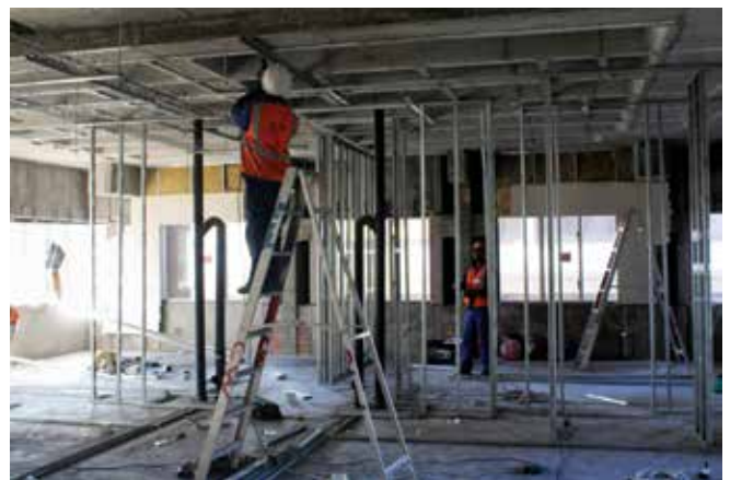
Murray & Roberts Western Cape has subcontracted all works related to the project, and has been tasked with managing these.
