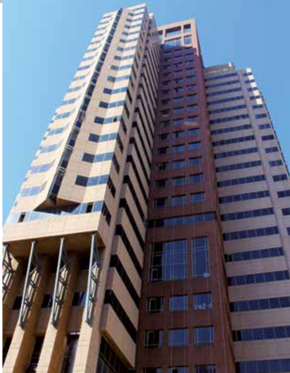
Murray & Roberts Western Cape is converting the first 11 storeys of the structure into a luxury hotel.
