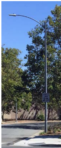
Figure 2-16: Roadway cobra head light fixture
