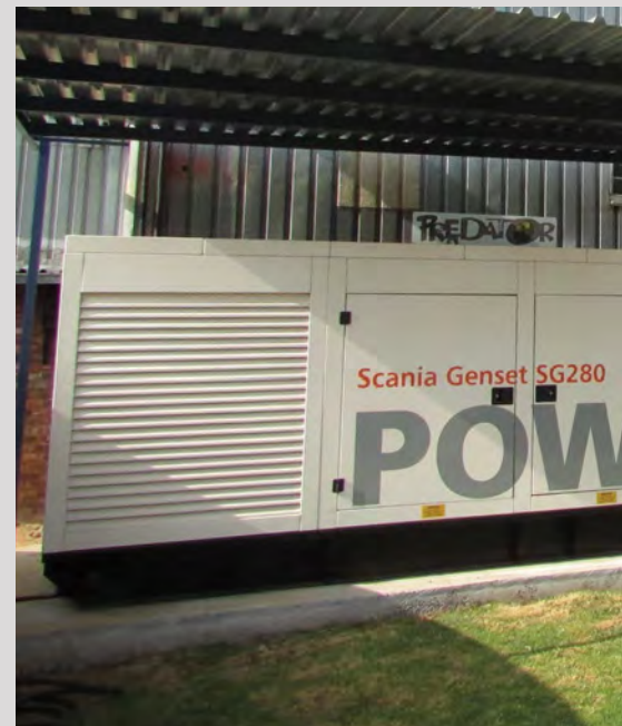
The Scania SG280 genset installed at Busco's manufacturing facility.
