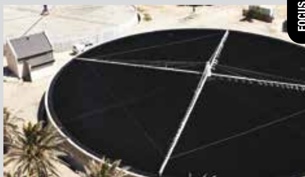
A similar trickling filter system utilising existing infrastructure, providing a cost-effective solution to increase water treatment capacity.
