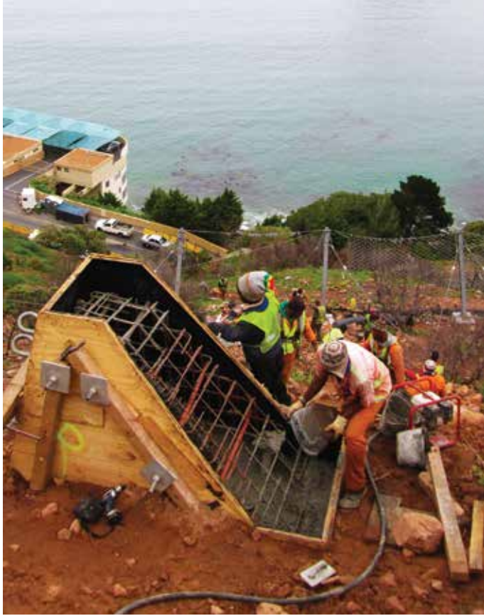
Debris in flow fence in northern gully.
