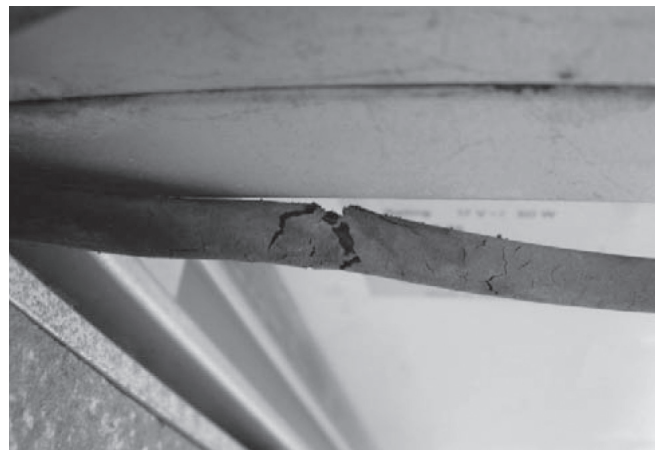
○ Figure 1: Wiring failures caused by ozone and high temperatures
