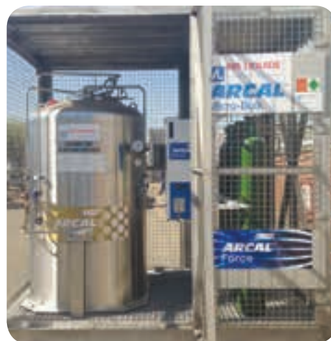
Air Liquide's patent-pending Arcal Micro-bulk onsite gas delivery system arrives tested and calibrated in a protective stainless steel container cage with a liquid argon tank, a dynamic mixer and a manifold of CO 2 cylinders.
