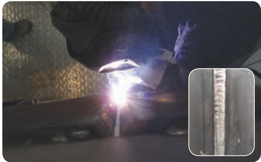
Manual shielded metal arc welding (SMAW) in the 3G position using UTP AF 6222 Mo PW and (right) a typical joint.
