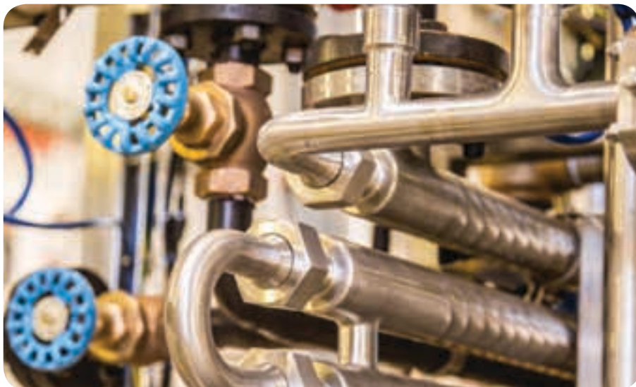
Plants generally comprise a closed system of tanks, heat exchangers, mixers, distillation columns and inter-connecting thin-walled pipes. Photo courtesy BOC and A&G Engineering.
