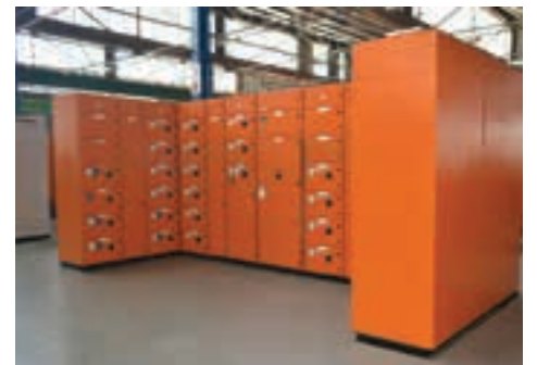
Motor Control Centres
