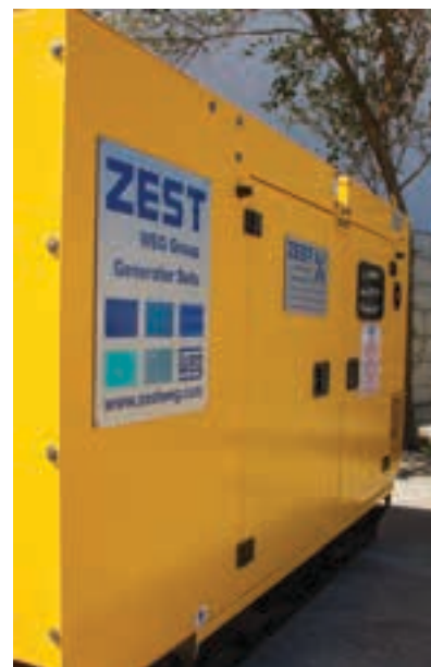
A 70 kVA, 400 V Zest WEG diesel generator set housed in a sound and weather proof enclosure.
