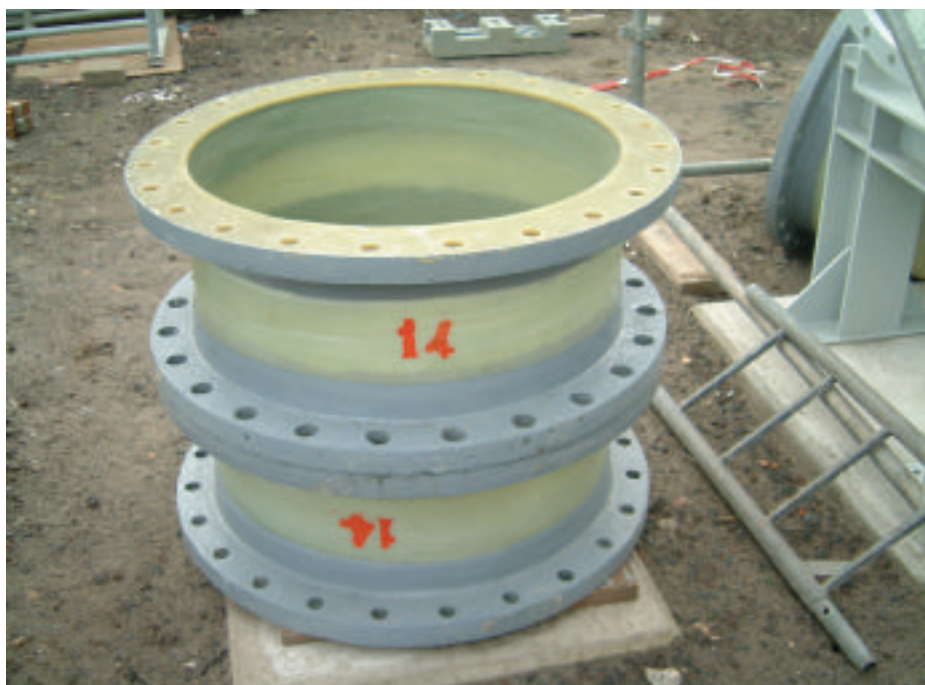
▼ Spool of a cooling water line: waste incineration in Rotterdam
