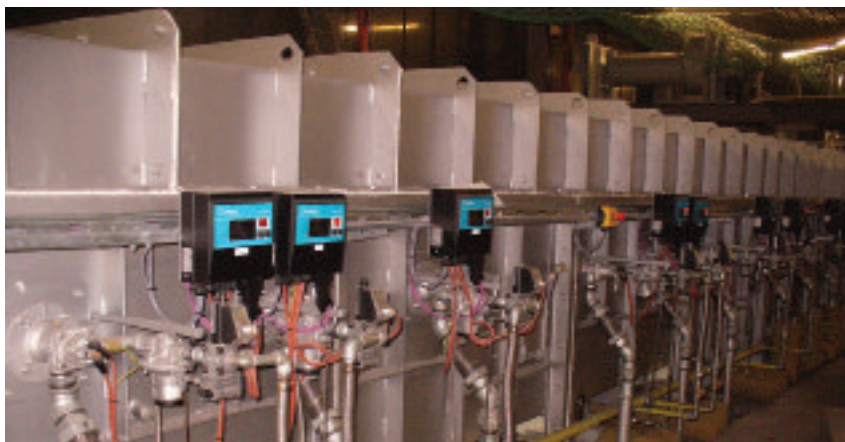
▲ Patenting furnace – side view
