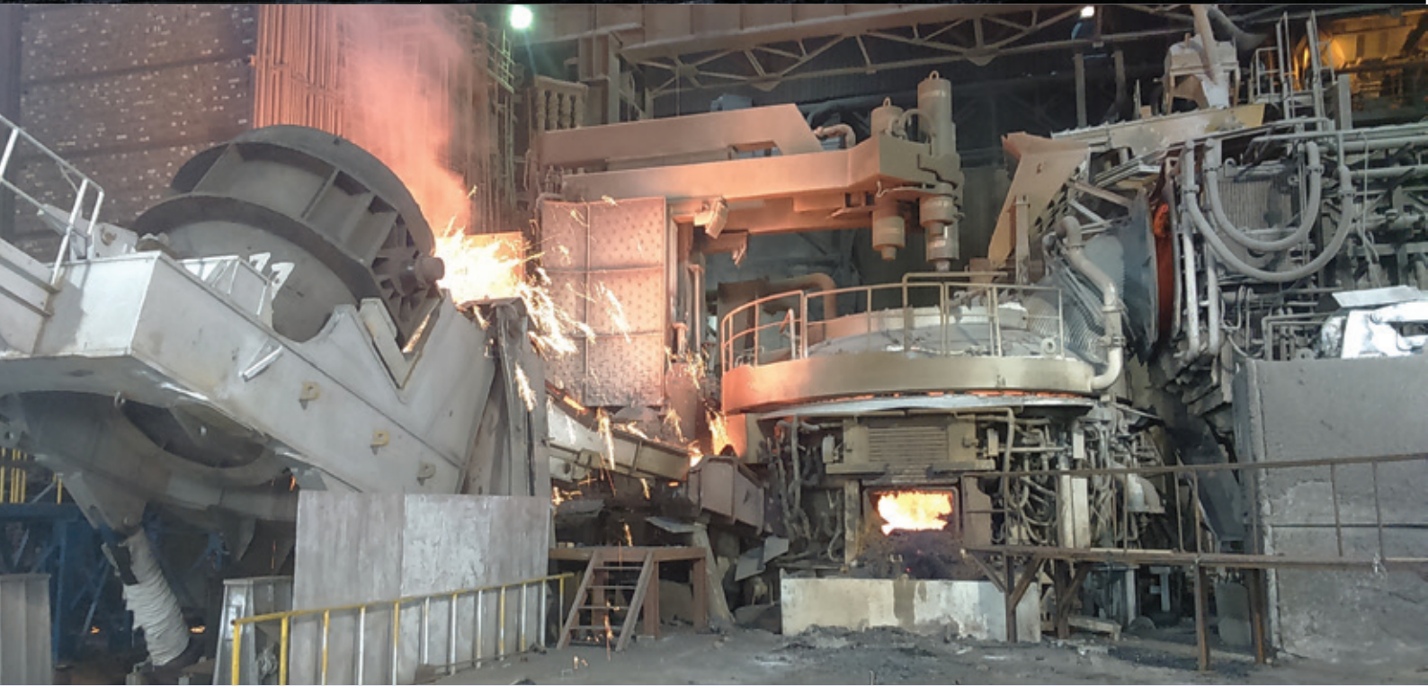
○ The new furnace at the Raigarh Steel Plant in India
