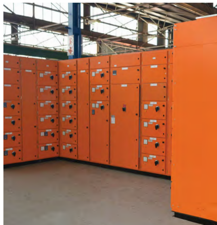
A fixed pattern MCC manufactured by Shaw Controls for an E-house destined for a mine tailings project. "There is no other manufacturer in the country that is able to manufacture everything in-house," says Van Niekerk.
