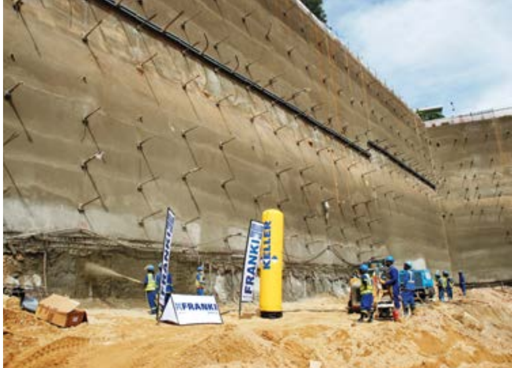
Gunite being applied to the trimmed face along the southern portion of the site.
