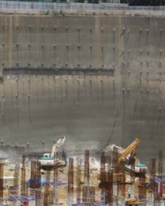
North western corner of the site where the excavation depth reached 32 m.
