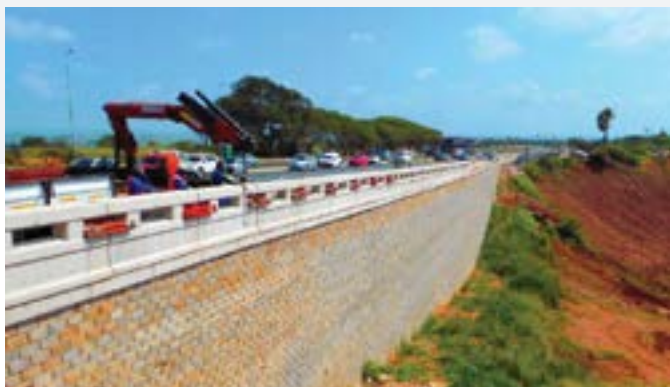
Installation of a crash barrier on the 11 m high Tensar TW1 wall at Ballito Drive.
