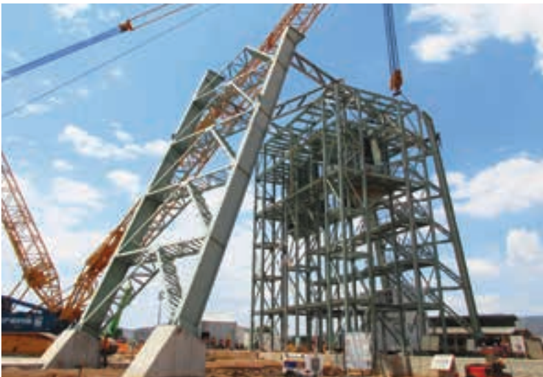
Photo taken during the erection of the headgear. A 600-ton capacity Demag crawler crane from Sarens was used to lift the heavy components.
