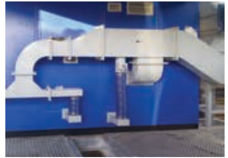
RTS Africa Engineering supplies inertial spin filters for the variable speed drive (VSD) panels typically used in large-scale mining projects such as the one pictured.
