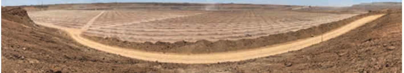
Block with 5 665 detonators in 2 683 blastholes ready for blasting using the AXXIS™ digital detonation system.
