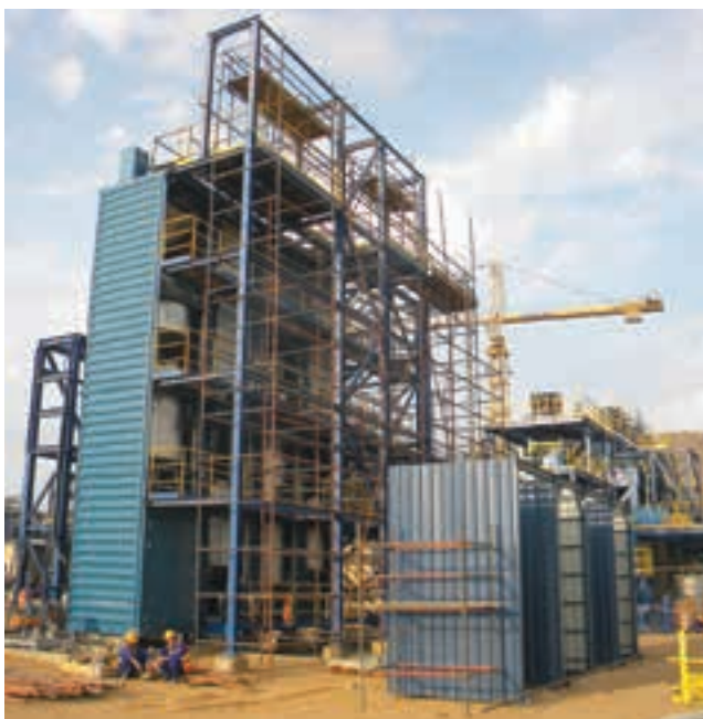
The zinc regrind facility at Bisha under construction in October 2015 (photo: Nevsun).
