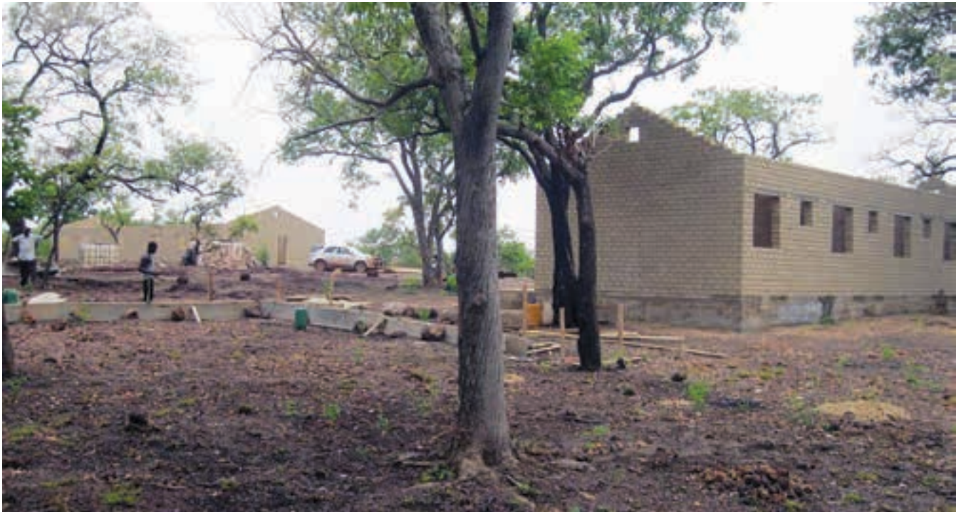
New accommodation modules serving the project.
