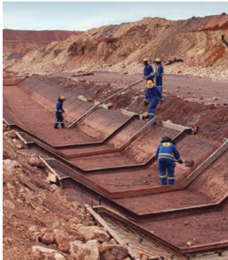
The concrete-lined canal is 4,6 km long, with the width of its base varying between 2 and 3 m.
