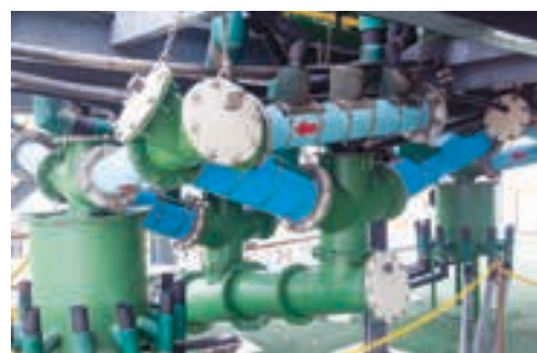
The cleaner concentrate and tail pipe launder arrangement, together with Multotec distributors.
