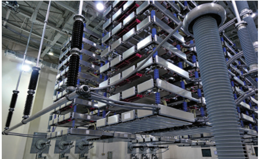
○ HVDC valves hall at Alstom
