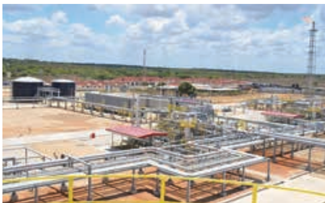
WorleyParsons was acknowledged by the former president of Tanzania for its 'valuable contribution to the successful completion ...' of the two natural gas processing plants at Madimba (Mnazi Bay, shown above) and Songo Songo Island.
