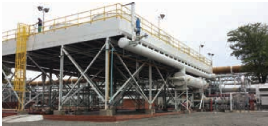
Vuselela's groundbreaking initiative uses waste heat from Anglo Platinum's ACP convertor cooling circuit to evaporate an organic liquid and drive an expansion turbine.
