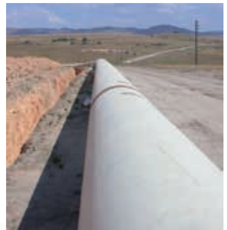
The Rompco Pipeline from Pande to Secunda built to bring gas to South Africa.
