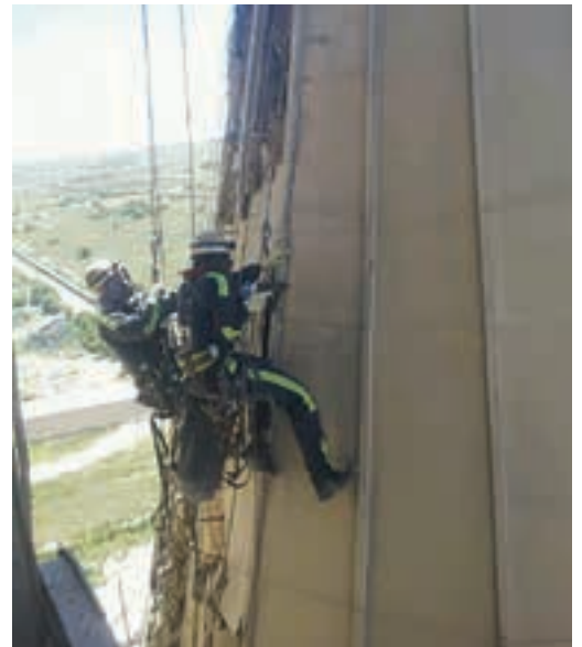
The inspection project was focused on the mill area of the cement factory.
