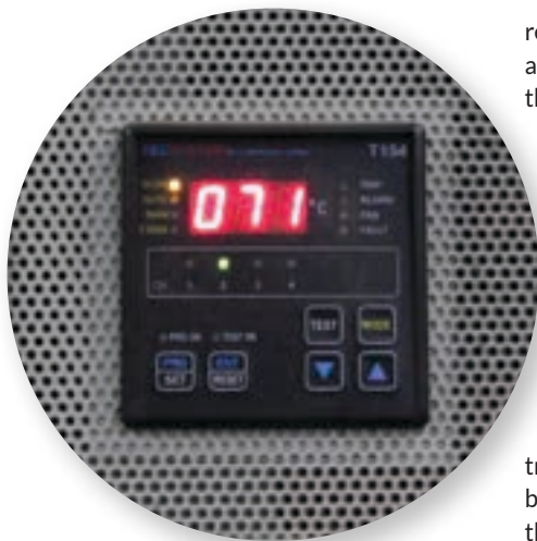
Pt100 temperature probes measure the temperature on each of the LV coils, and a temperature controller designed for cast resin transformers manages the fans and alarm and trip alerts.
