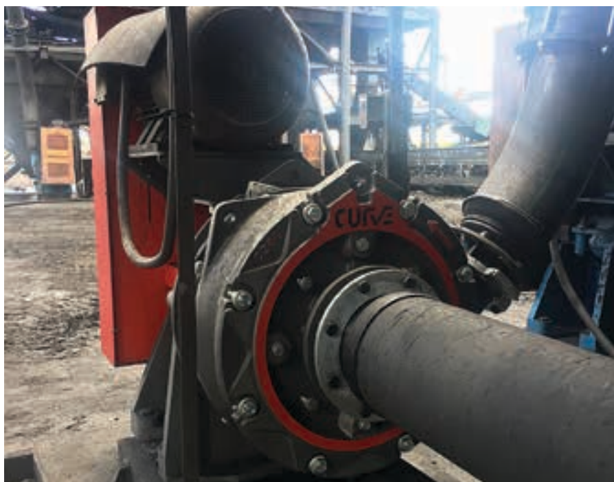
Hernic Ferrochrome is currently retrofitting the pumps at its OB-Plant with Curve S150s from Pump and Abrasion Technologies.
