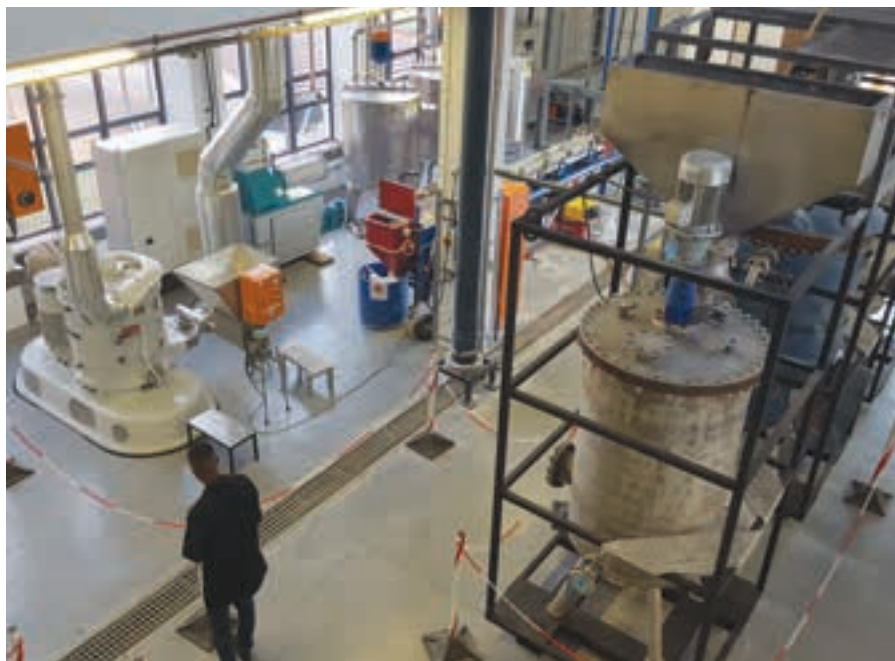
The chemical processing plant is equipped with high temperature and pressure chemical reactors, process tanks, a filter press, dryers and a bag house.
