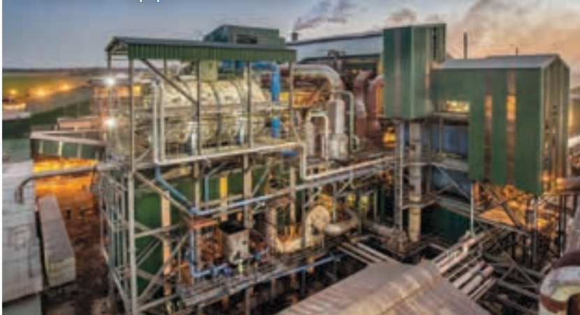
Bosch Projects' continuous vacuum pan supplied into Zambia's Nakambala Product Alignment and Refinery project.
