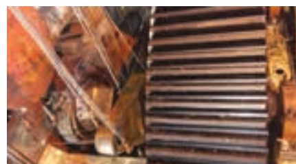
BMG's KZN field service team has been involved in a number of field service projects in the local sugar industry during recent off crop seasons, as well as dealing with urgent breakdowns in sugar mills and refineries.
