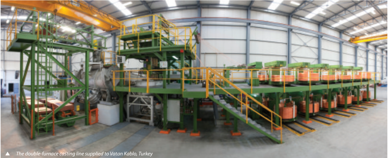
▲ The double-furnace casting line supplied to Vatan Kablo, Turkey
