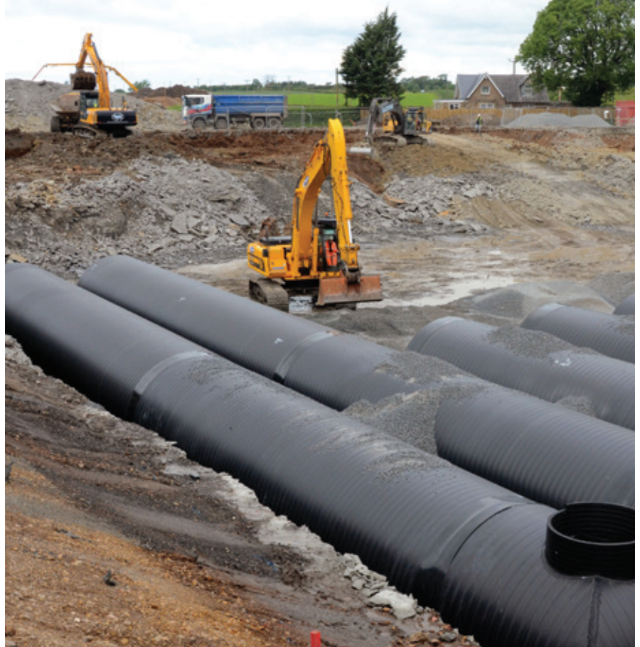
This 10,000m 3 storm water detention tank project in Scotland consists of DN/ID 2.6m Weholite pipes
