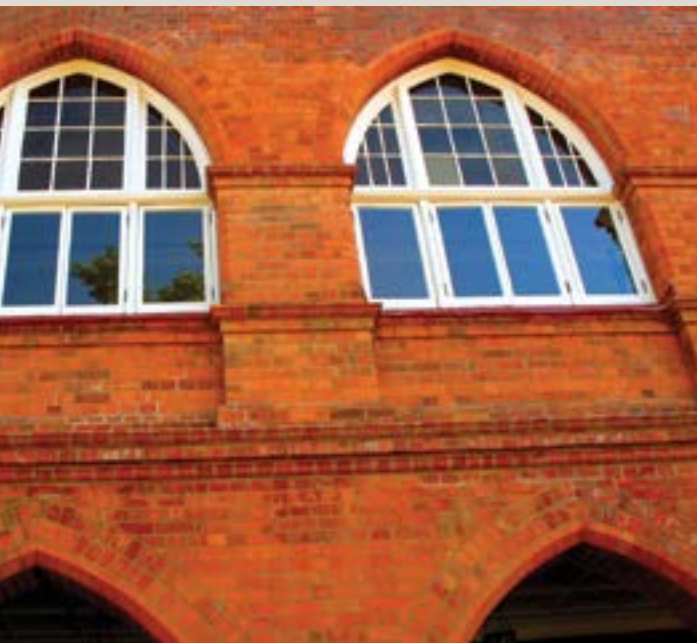
Photograph of windows which are arched, and framed by special shaped bricks, also showing the detail of special shapes used on horizontal courses in the style of the period.
