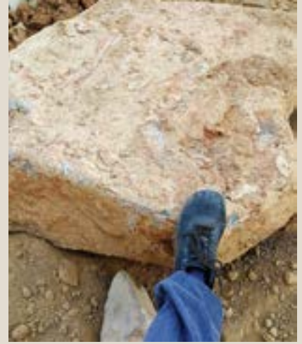
A photograph showing a typical underground boulder that made the foundation excavations a formidable task.
