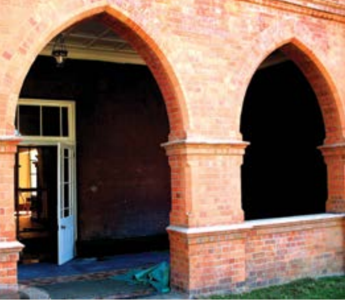
The arched wall surrounding the veranda along the side of the building, showing the detail of the special shaped bricks. Bricks made at Corobrik's Midrand factory were used where individual bricks had to be replaced in order to preserve the original look of the brick work.
