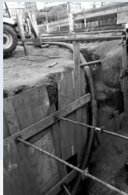
Pulling the new HDPE pipe (for the HDD line perpendicular to the tracks) into the drilled hole.
