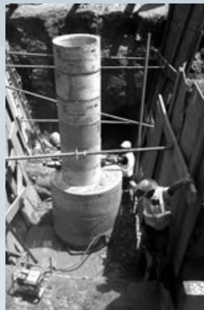
Construction of a new sewer manhole in-between the railway tracks at Park Station in the Johannesburg CBD.
