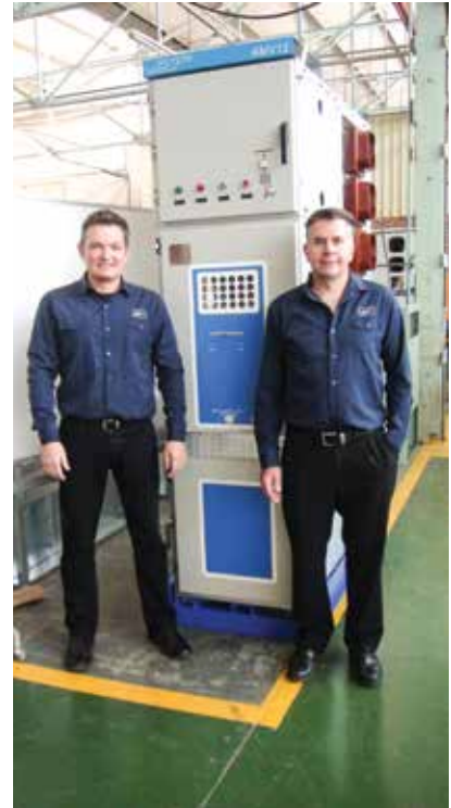
ACTOM MV Switchgear's Rhett Kelly (left) and Greg Whyte pose in the business unit's Knights plant with a compact AMV12 unit.
