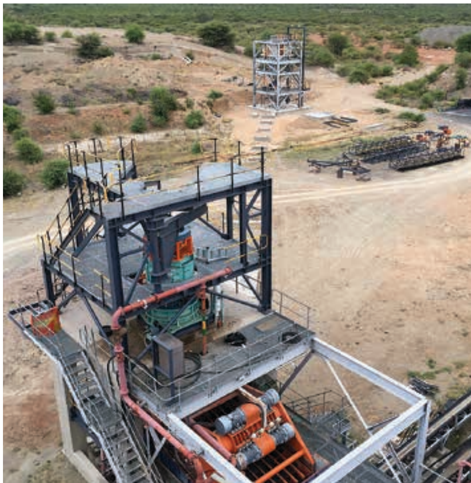
The new Kawasaki secondary cone crusher (foreground) with the relocated surge bin and conveyor plinths in the background (photo: Kimberley Diamonds).
