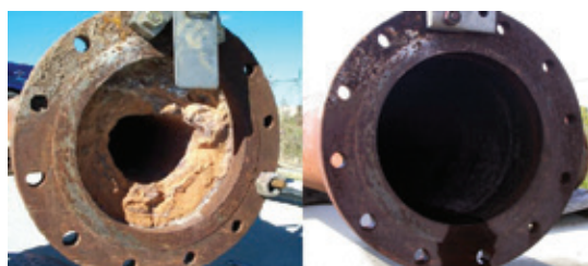
Before and after: Pipetech uses high-pressure water technology to remove scale and debris from tubes, pipes and process equipment
