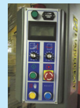
PLC Control With LCD Display
