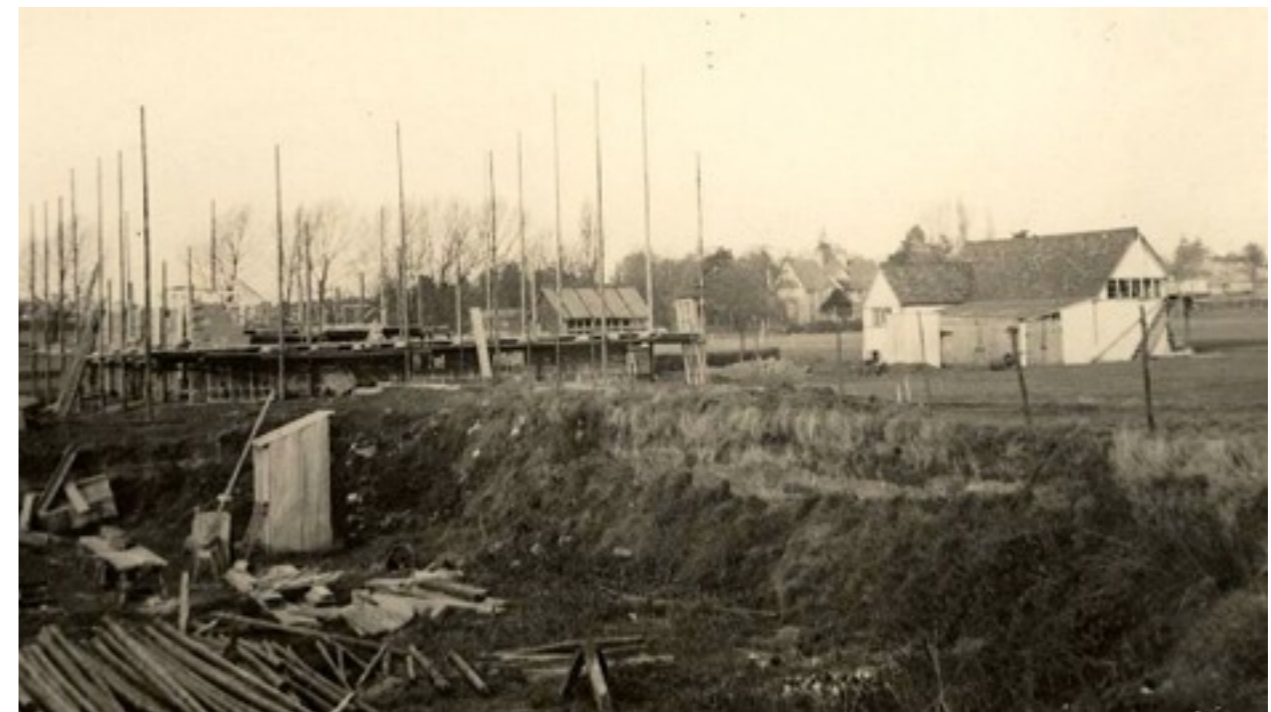
THE ERECTION OF THE 1933 CRICKET PAVILION IN THE FOREGROUND WITH ITS 1922 PREDECESSOR TO THE RIGHT
