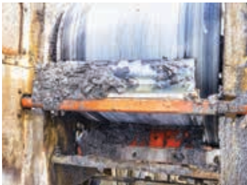
The carryback had the consistency of toothpaste, adhering chunks of aggregate to the belt and causing damage to pulleys and headers.
