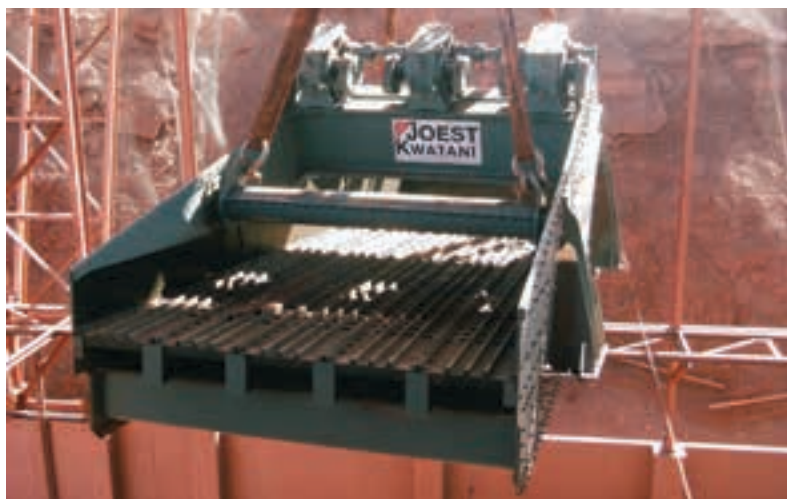
A Joest Kwatani 53-ton exciter driven scalping screen being installed at an iron ore mine.
