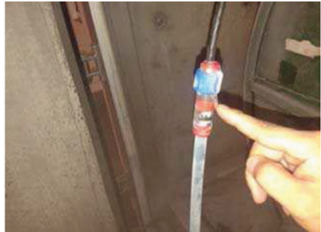
○ Figure 5: Water frozen around end caps
