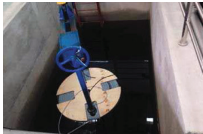
○ Figure 1: Micro-duct with cable soaked in water
