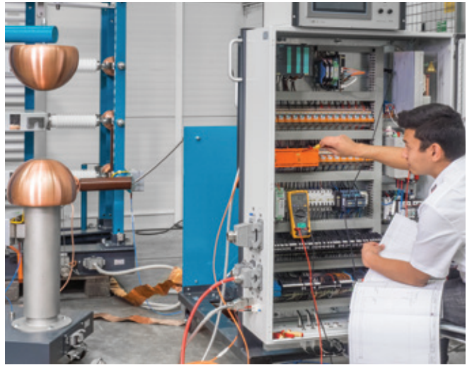
○ The high quality of the services is ensured by the continued training of service employees in Dresden by Highvolt, like Alex Bernardi, pictured, and by teaching on new product developments
