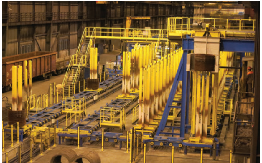
○ The new wire handling system at Swiss Steel
