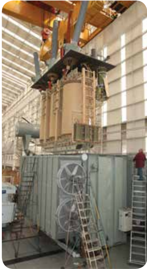
Seen in ACTOM Power Transformers' Wadeville, Germiston plant is a core and winding assembly being lowered into the tank of a large 315 MVA 275 kV power transformer similar to those on order for City Power's new Sebenza intake substation.
