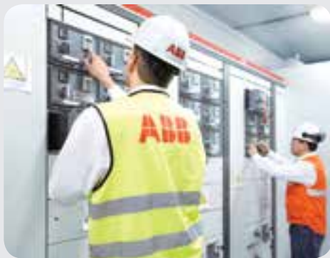
MNS contributes to a safe maintenance environment.
